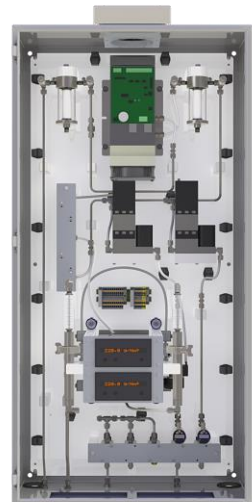
Ozone Generation Panel
